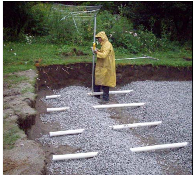
The tiles of new septic system bed are being surrounded by sand and gravel.
