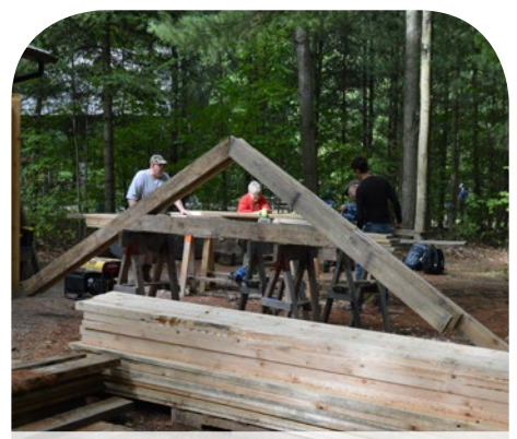
Volunteers help build a shed using Pioneer building methods at the Historic Fort Willow Conservation Area to further replicate the War of 1812 at the site.
